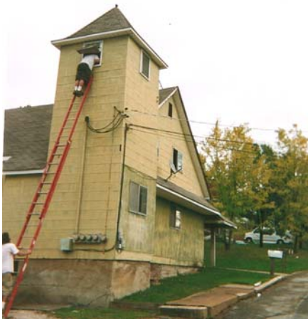
Demolition crew members check to see if tower bell is still in place at Circle Street structure.
